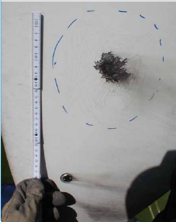
Figure 18 Example of Damage Caused by Lightning [22]
