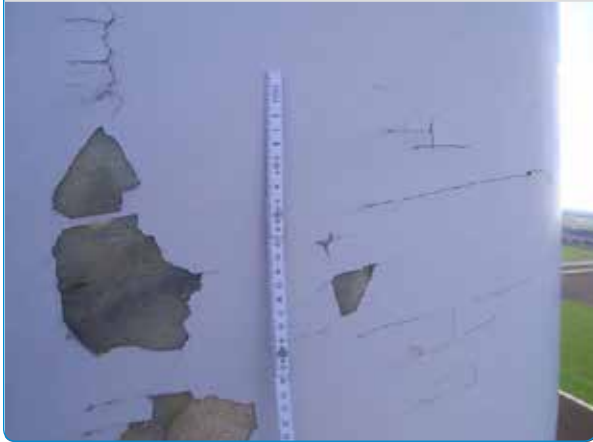
Figure 15 Cracks and Flaking in Gelcoat [22]
