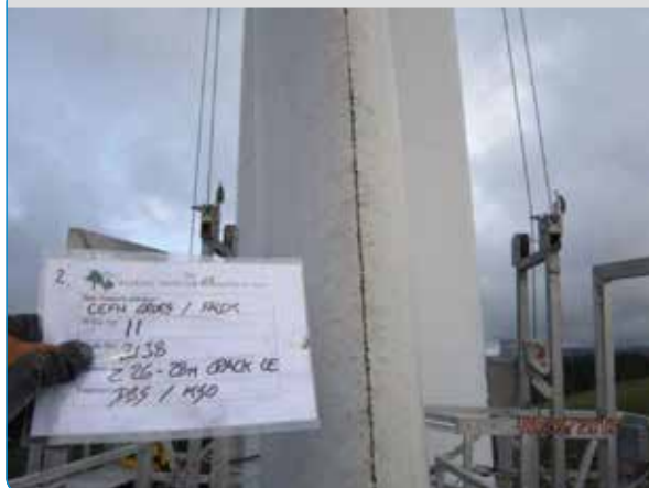
Figure 14 Cracks in Adhesive Bonding [21]
